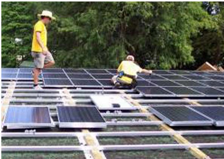
Installing Evergreen Solar panels on a National Park Service building at the White House
